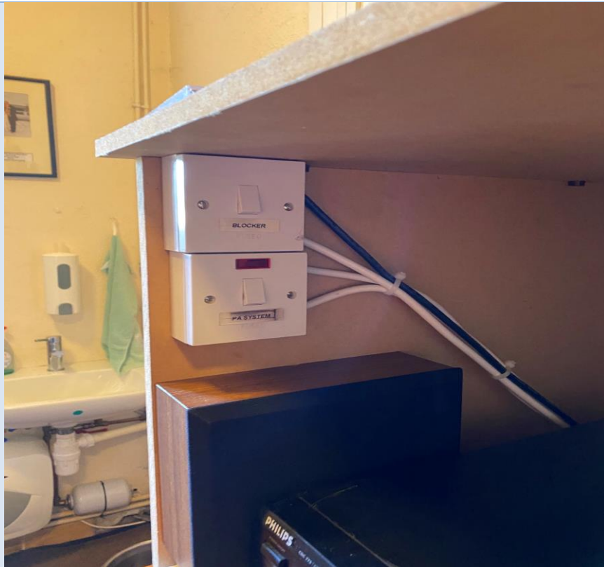
Figure 11 Wired back to control switch
