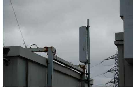
Telemetry outstation antenna in Western Power Distribution’s 400 MHz LTE trial in Bristol, UK
