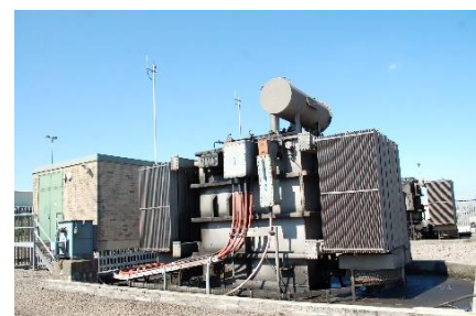
Unlike consumer products, utility assets are often designed with a service life of up to 50 years.
