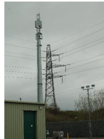
Western Power Distribution's 400 MHz LTE trial base station at an electricity substation near Bristol in UK
