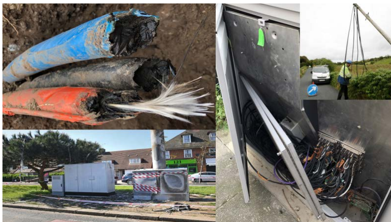
Figure 5: Plant Damage, including Arson, Vandalism and Theft
