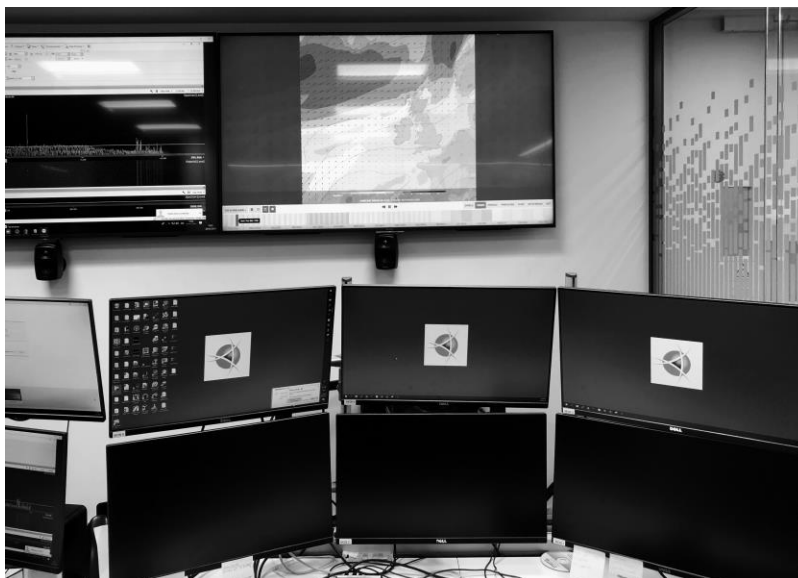
Figure 1: ComReg Monitoring Room at Dockland Central
