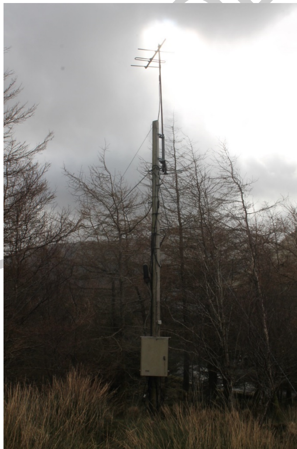
Figure A.2: Radio Installation at Customer 3 property location
